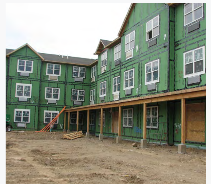
Progress is made on construction of new low-income senior, special needs, and veterans housing in Upper Saddle River.
